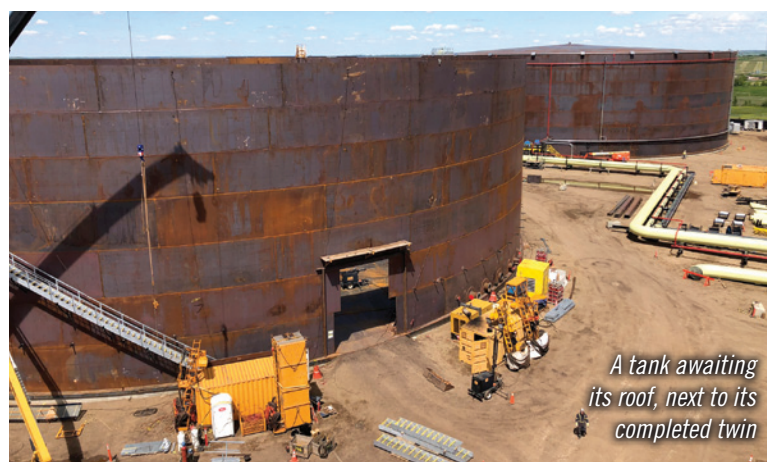
A crane within one of the half-finished tanks highlights the scale of the job.
